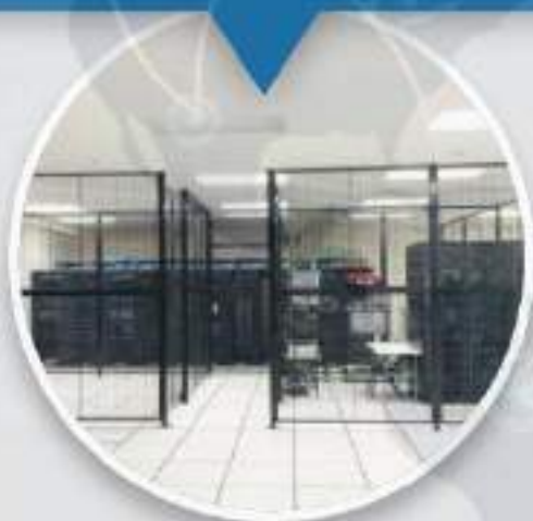
DATA CENTER TIER 3
